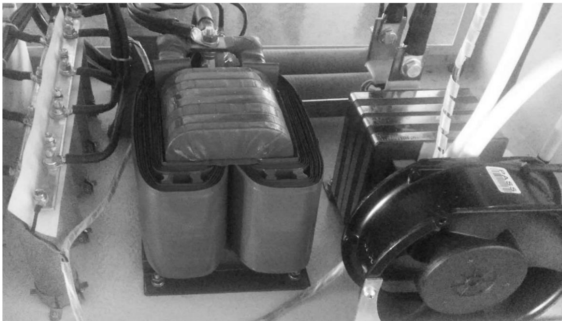
10.5 Output Filtering Capacitor and DC choke
